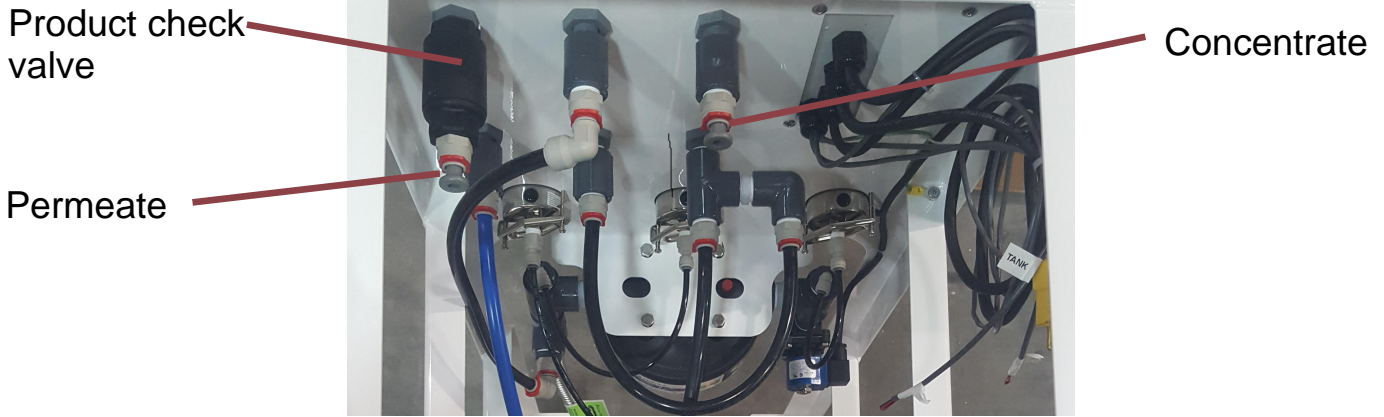
System rear view
